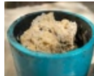
FOG IN PIPE
